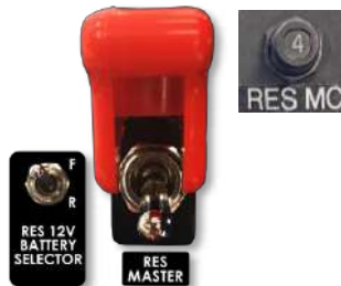
Figure 8 Guarded RES master switch, battery selector switch and RES MC circuit breaker
