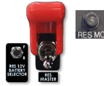
Figure 7-25 Guarded RES master switch, battery selector switch and RES Motor Controller (MC) circuit breaker
